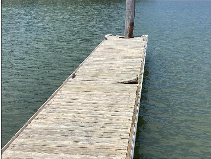
Photo #13: Some boards have warped and require replacement.
