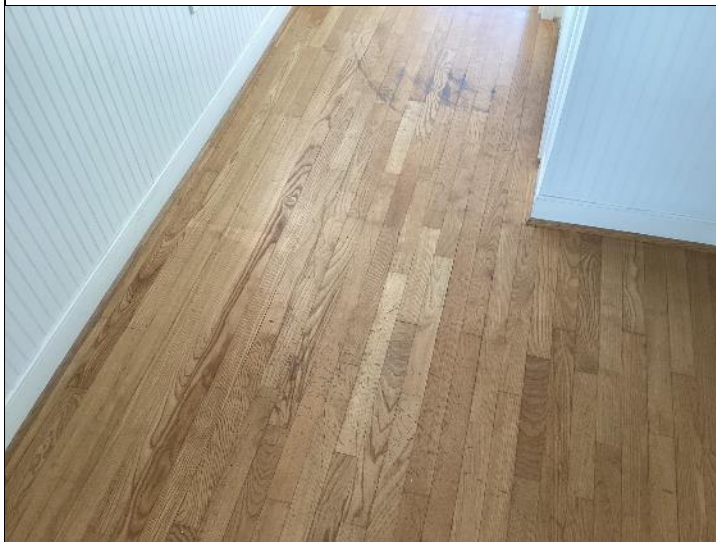
Photo #23: The hardwood flooring should be refinished on a cyclical basis.
