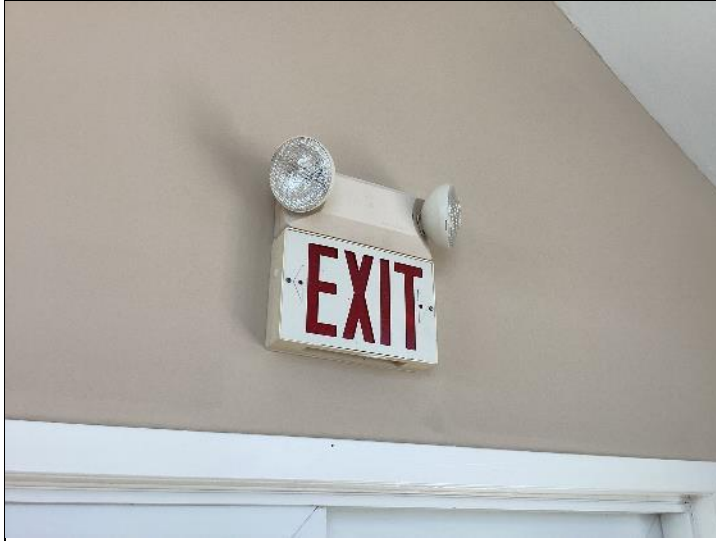
Photo #31: Some exit lights were inoperable during our review. We recommend they be tested and replaced where needed.
