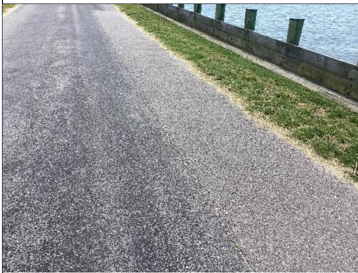
Photo #15: The asphalt was in poor condition during our review. We recommend cracks be maintained sealed to prevent displacement of the subbase.
