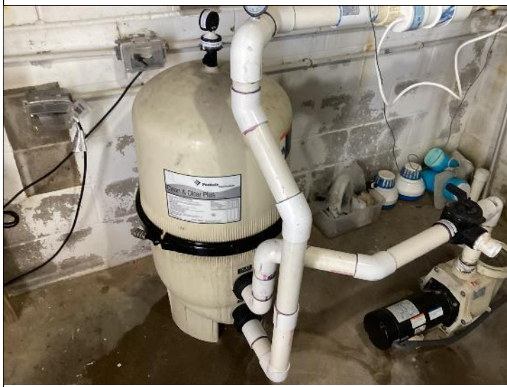
Photo #48: Pool filter and pump.
