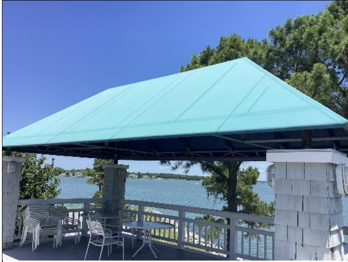
Photo #40: The awning has faded, but otherwise presented in acceptable condition.
