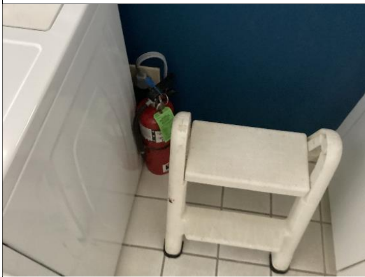
Photo #27: Fire extinguishers are required to properly mounted per fire code regulations.
