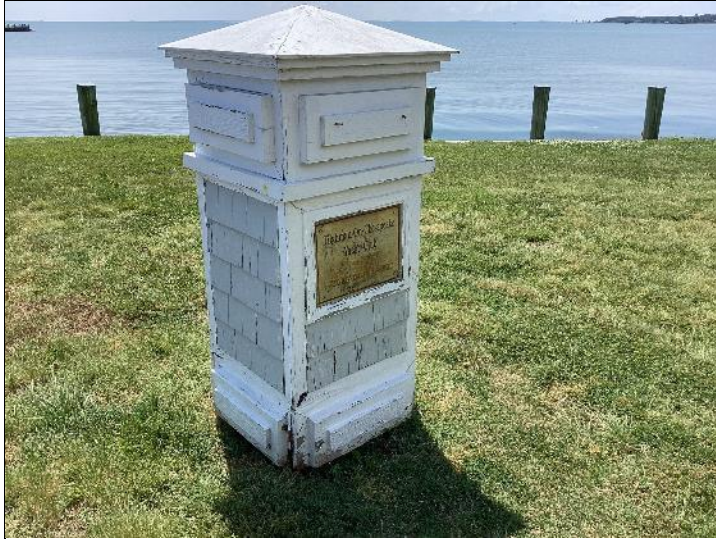
Photo #7: We recommend the entry columns be reconditioned.
