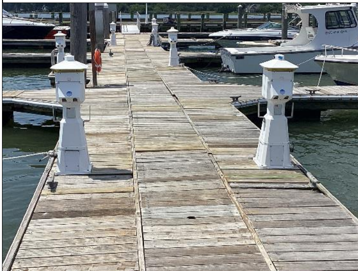
Photo #14: Deteriorated boards should be replaced where needed.
