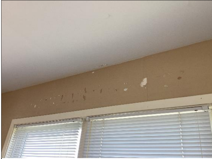
Photo #25: Damages noted to some of the interior wall finishes. Consideration should be given to repainting these areas.
