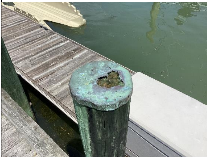
Photo #2: Some of the piling caps have deteriorated and should be considered for replacement to help preserve the wood.
