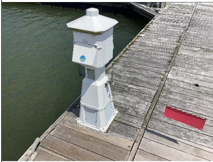
Photo #12: Dock power pedestal.
