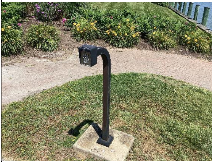
Photo #6: Entry gate arm keypad. We recommend the metal post be properly prepared and painted to preserve the metalwork.
