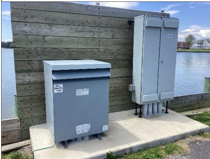
Photo #17: Site transformer.
