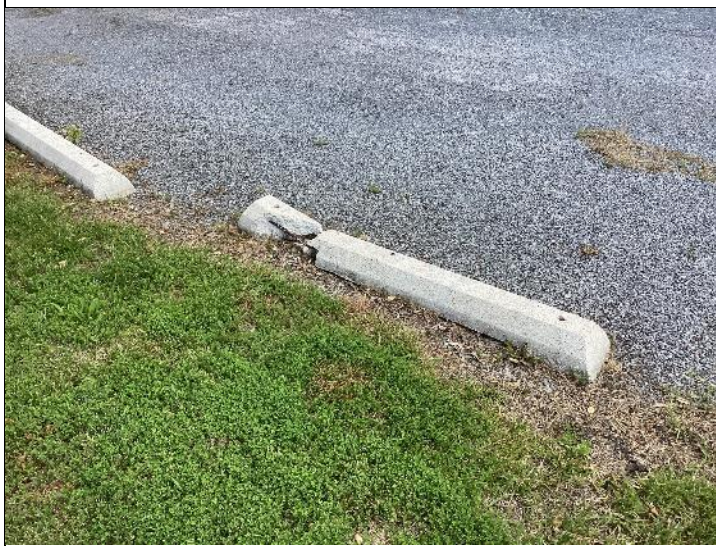
Photo #18: Damaged concrete wheel stop.
