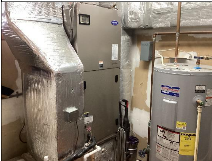
Photo #29: HVAC and water heater servicing the community building.
