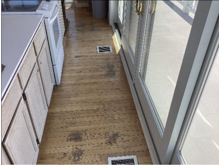
Photo #34: The hardwood flooring should be refinished on a cyclical basis.
