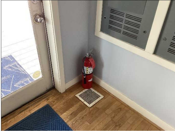
Photo #28: Fire extinguishers are required to properly mounted per fire code regulations.
