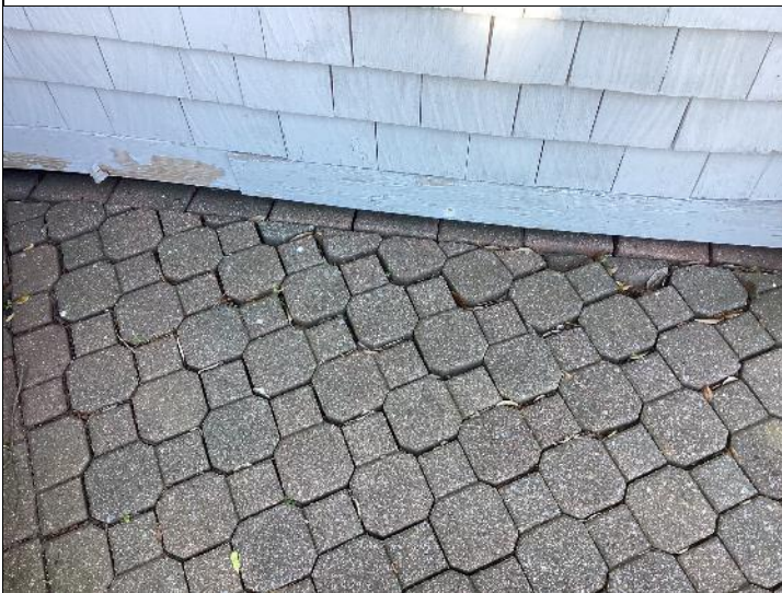
Photo #20: Some of the pavers have begun to settle and separate. Consideration should be given to applying a fine sand to the openings to help hold the walk together.
