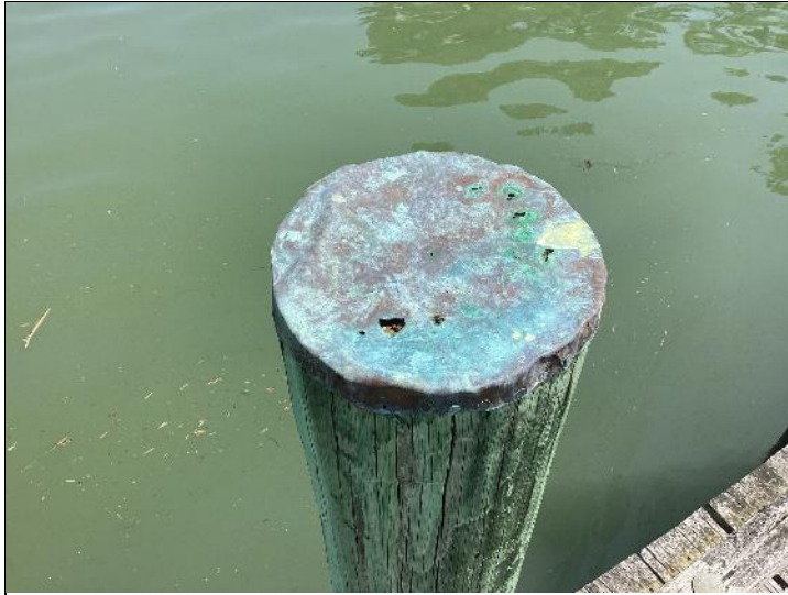
Photo #1: Some of the piling caps have deteriorated and should be considered for replacement to help preserve the wood.
