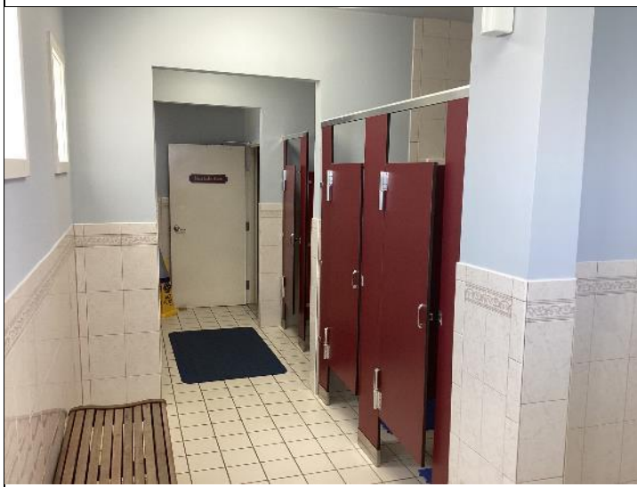
Photo #30: Typical bathroom finishes. The bathrooms presented in good condition during our review.
