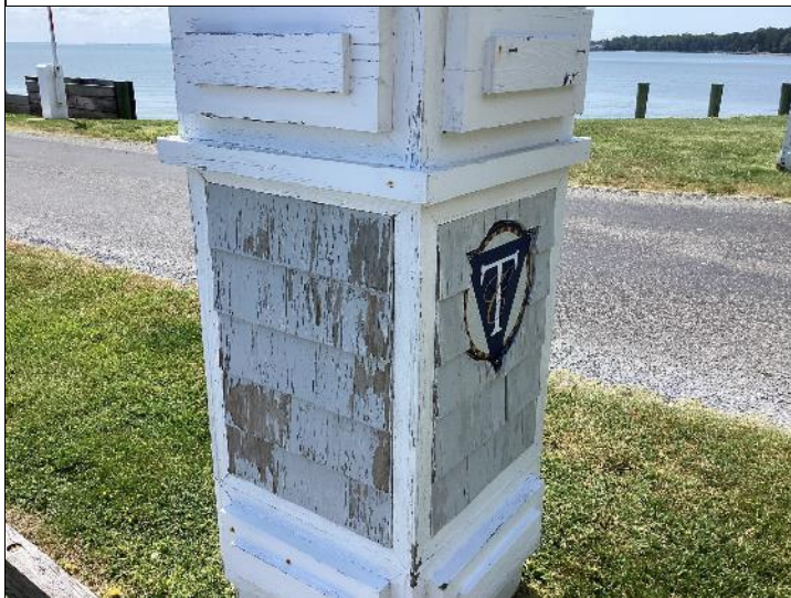
Photo #5: We recommend the entry columns be reconditioned.
