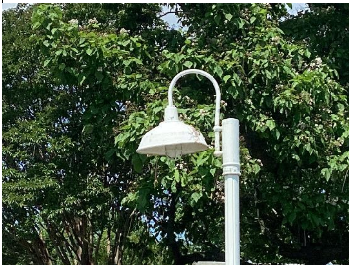
Photo #3: Typical pole light.
