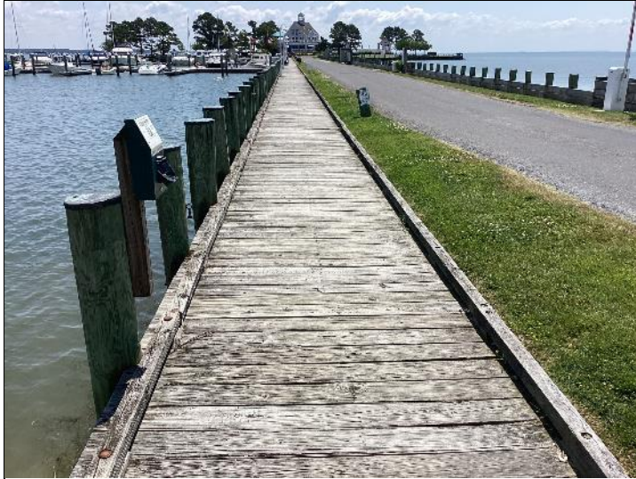
Photo #4: Boardwalk. Consideration should be given to sealing the decking with a wood preservative to help make it last.
