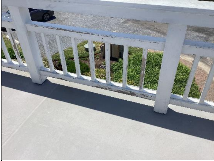
Photo #37: We recommend the railings be properly prepared and painted.
