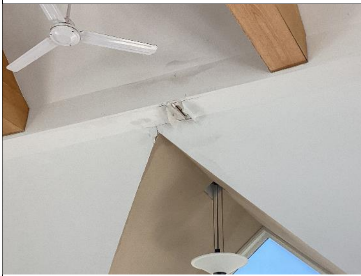
Photo #33: Apparent water damage was noted in the ceiling of the community building. We recommend this be monitored and repaired accordingly.
