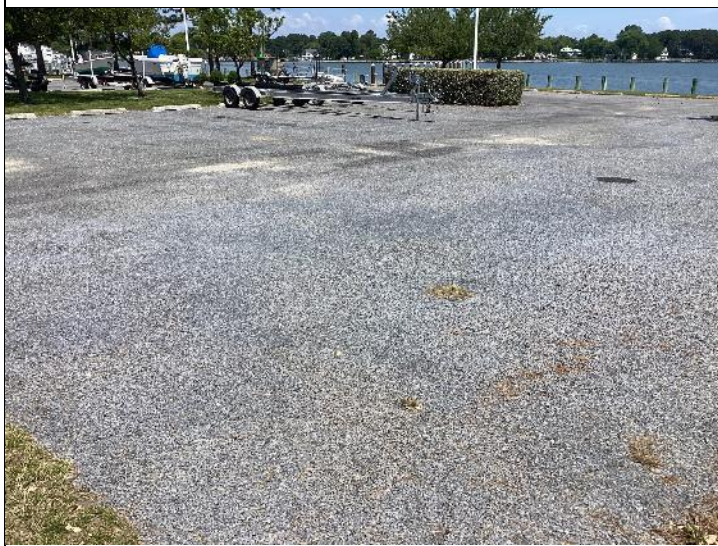
Photo #54: The asphalt should be considered for repaving.
