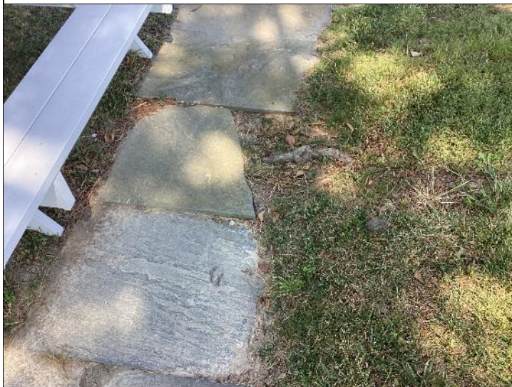
Photo #53: Damaged steppingstone paver.
