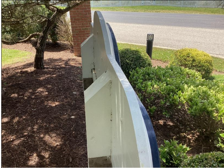
Photo #4: The entry monument appeared to be in good condition during our review.
