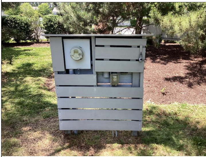
Photo #6: Electrical metering and switchgear servicing the entry lighting.
