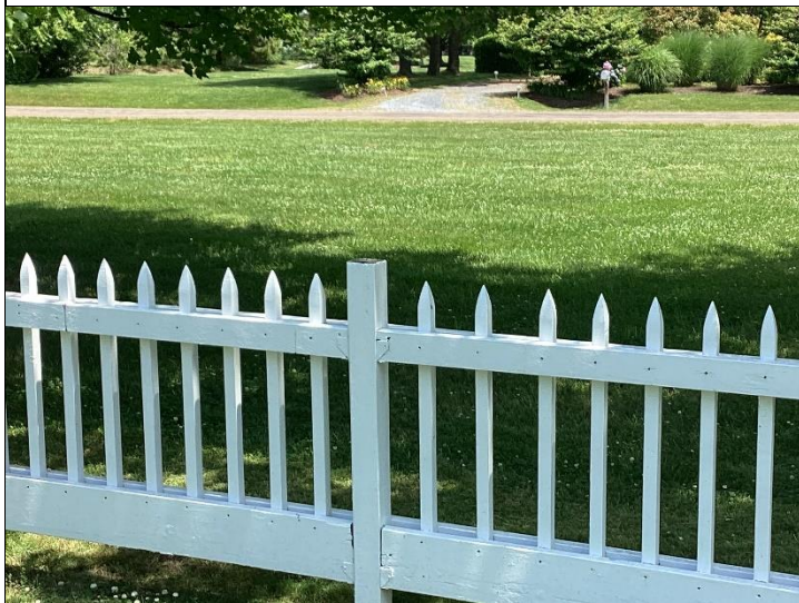
Photo #5: Some fence post caps were missing. We recommend these be replaced where needed to prevent excessive rainwater intrusion and possible damages during freeze/thaw cycles.
