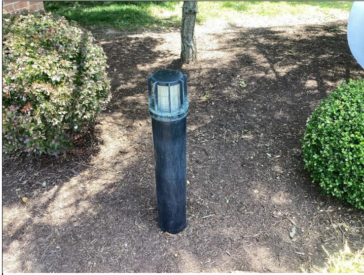
Photo #1: Landscape bollard lighting at entry.
